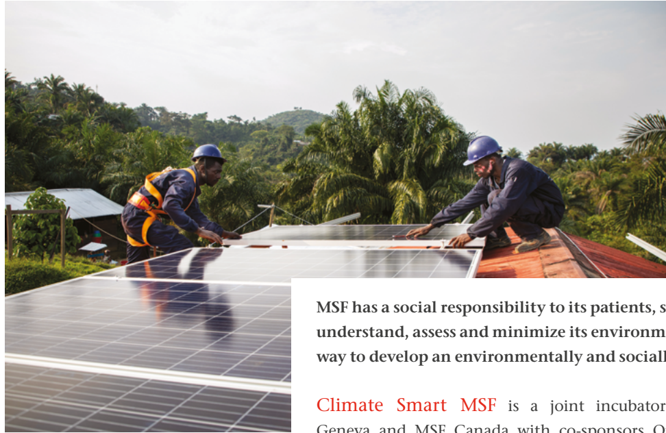
MSF has settled a solar panel system at the General Hospital of Kigulube in Sud Kivu (Democratic Republic of Congo) to give autonomy to the health structure for the next 20 years.
